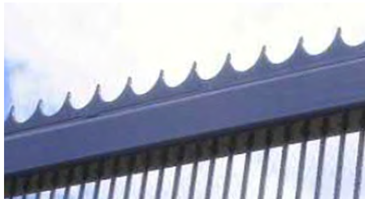
Above: Extract taken from the submitted design and access statement showing the indicative serrated topping to the proposed boundary fencing.
